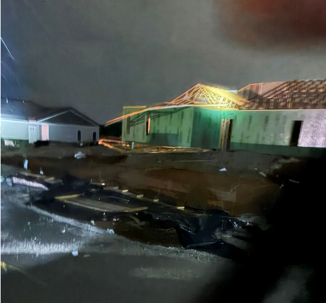
Damage to Savannah of Pikes Creek Construction site
