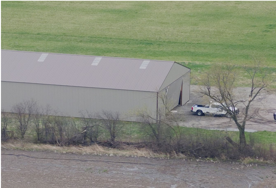
Barn Door Damage
