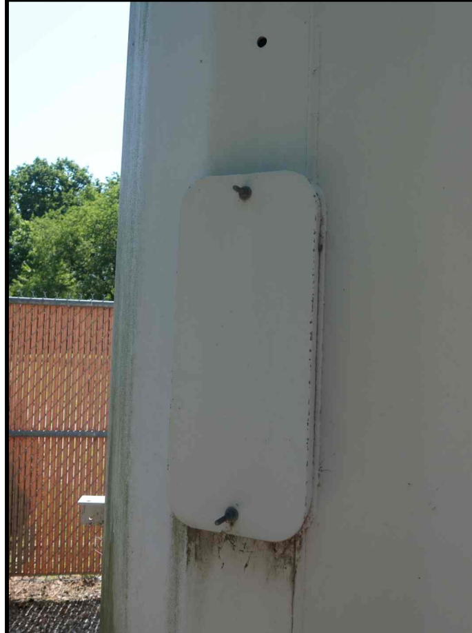
D LOWER TOWER COAX PORT(S)
