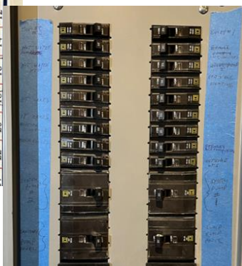
▲ Figure 2 Emergency Panel in Boiler Room Near Village Hall
