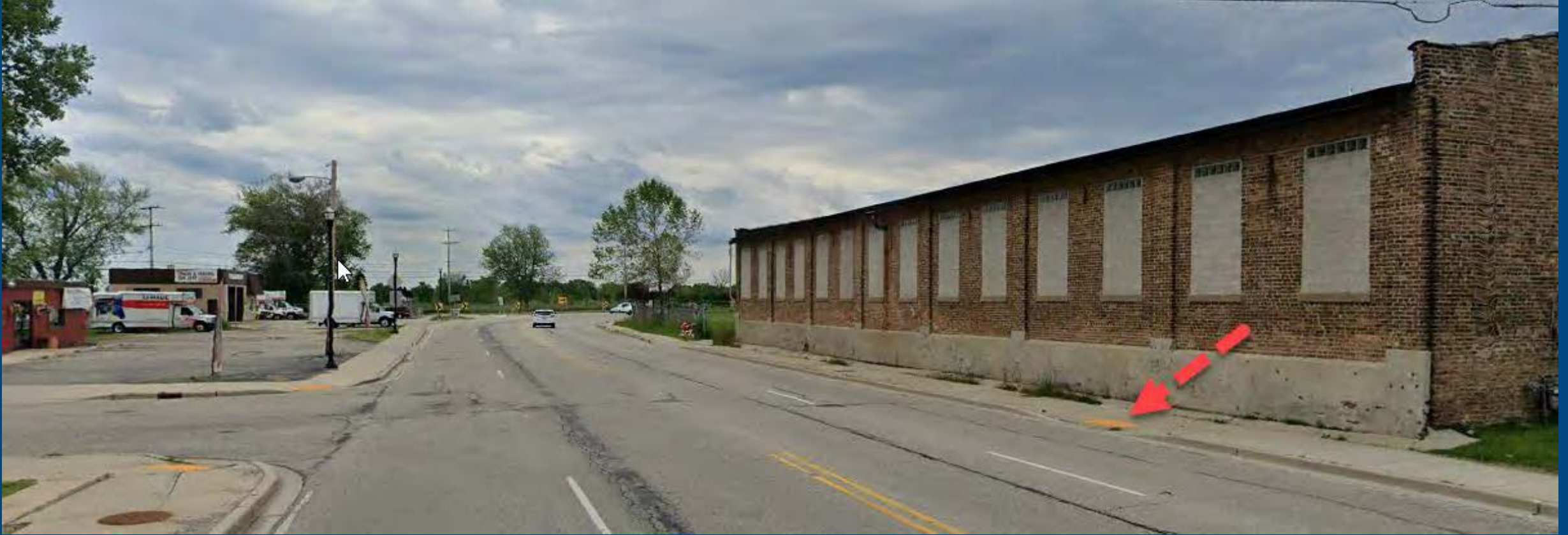
Intersection of WIS 32/24 th St. : Curb ramps do not line up.
