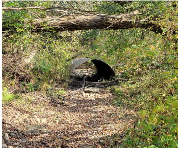
Figure 5. This culvert at Station 0+90 has lost the surrounding backfill and road surface, but remains in place.
